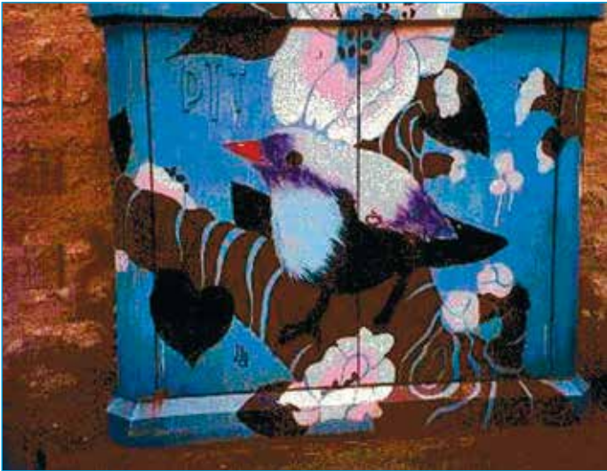
Telephone control box, Perigueux, France. Photograph reproduced with the kind permission of Richard Lucas.
