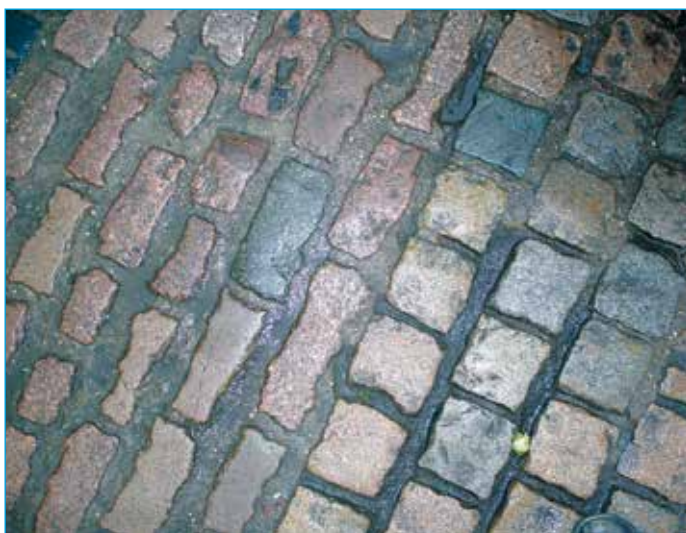
Natural stone setts used in the area of Boston Market Place, within the Conservation Area (See section 4.3.6 Materials).
