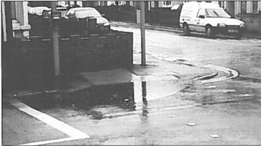
A poorly constructed drop-kerb crossing point leads to localised flooding.
